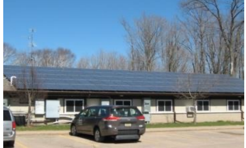
Solar PV on the Forest County Potawatomi assisted care building, a project completed using a tax equity partnership.
